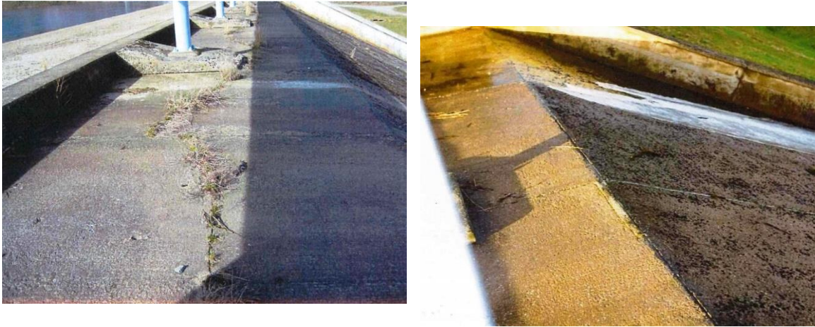
Figure. B5 Historic crest cracking and isolated seepages on the left side on the chute
