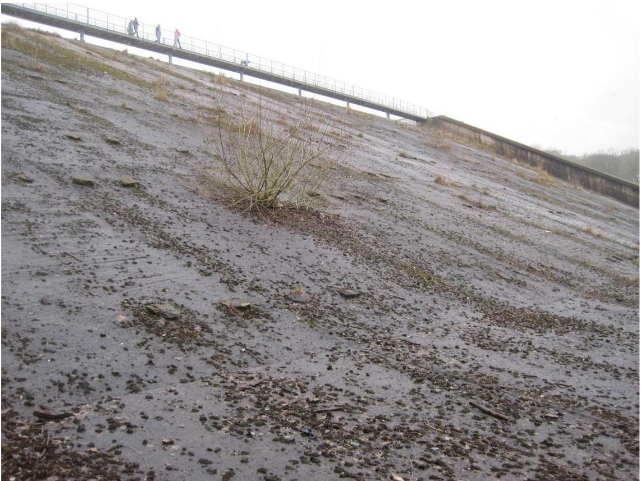
Figure 10. Evidence of Poor Maintenance with Vegetation and Saplings Growing in Joints, January 2018
