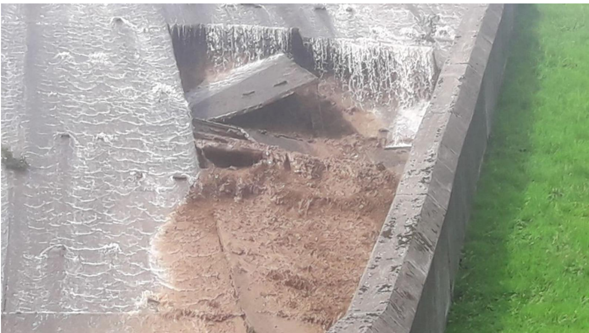
Figure 6. Four Sections of Panels Collapsed into the Void
