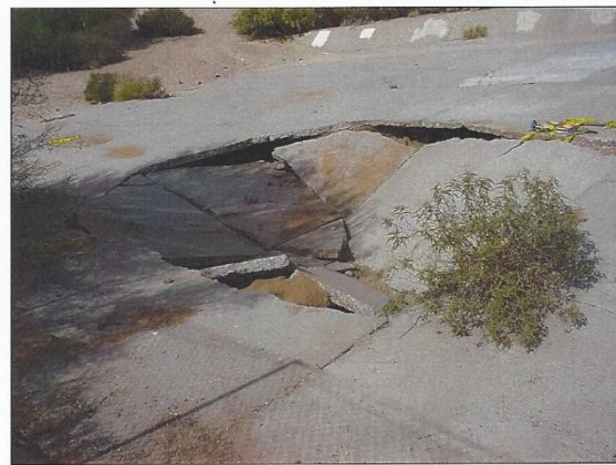
Figure 4.—Structural collapse of the slab system occurs when enough undermining has occurred to cause loss of support. This damage is typical of slabs placed on soil foundations (note: this slab is not reinforced so failure is more evident).
