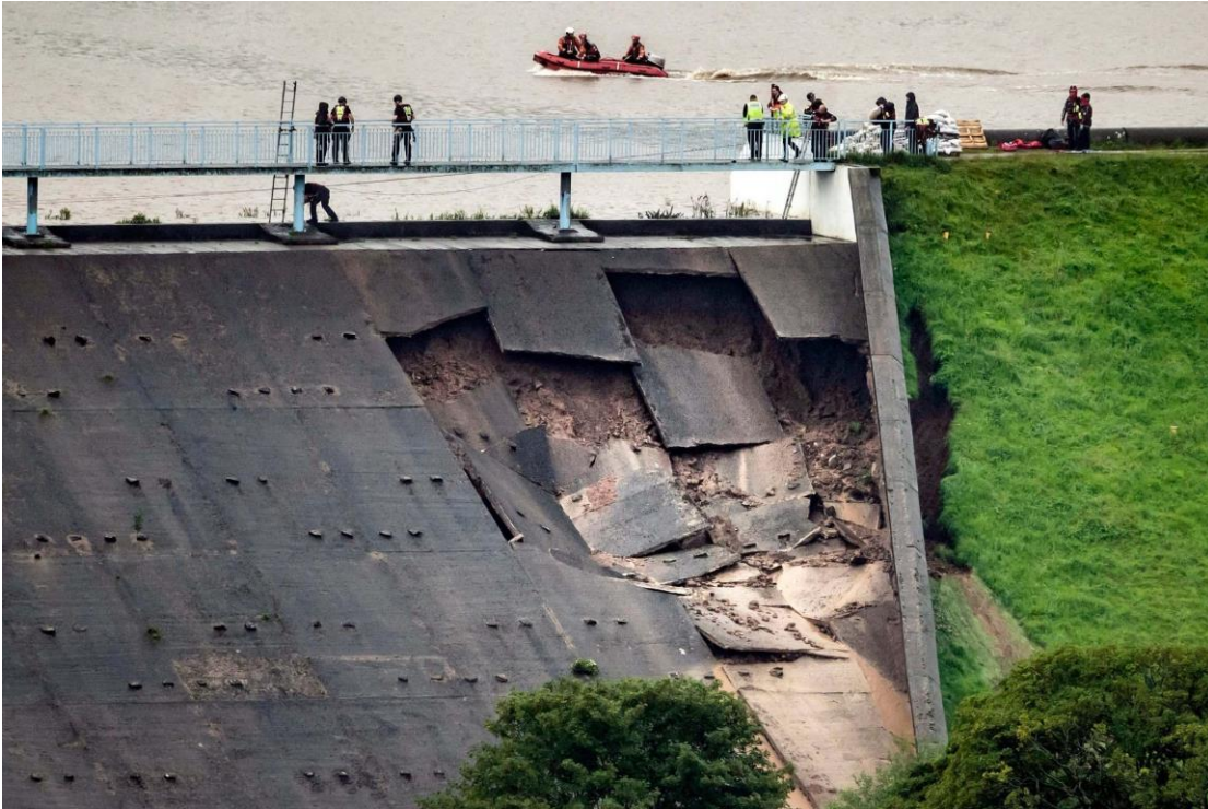
Figure 7. The Final Stage of Collapse of Panels. Note the undermining of the left-hand chute wall.
