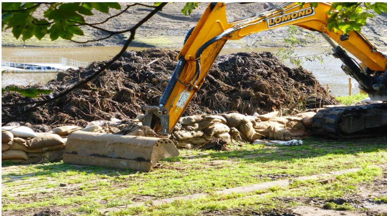
Photo GA8. Here are the many tonnes of mud, weed and stone that had to be cleared from the convergence basin immediately in the crisis, critical to saving Whaley Bridge from considerable destruction. It illustrates the huge loss of capacity and the undeniable systemic neglect of routine maintenance at Toddbrook in all the channels and culverts which are fundamental to the effectiveness and safety of the system. ( see GA2 many other photos)
