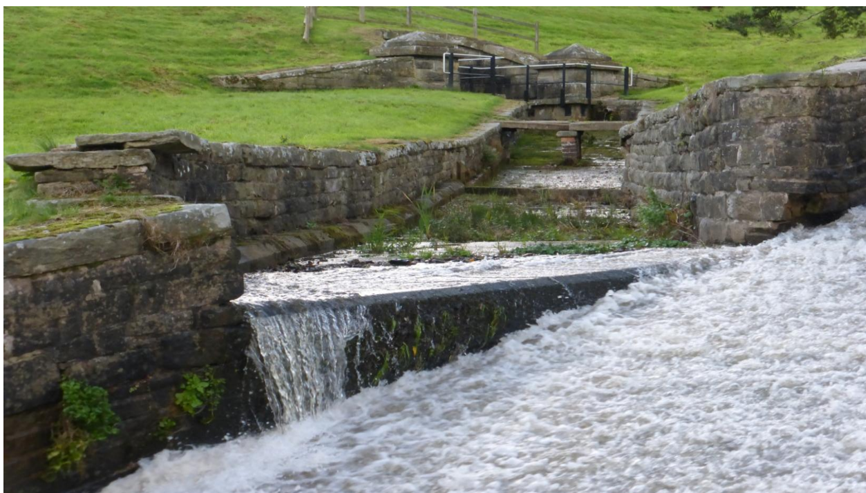
Photo GA9. The discharge culvert for Valve 1 into the Bypass provides a clear demonstration of the Primary Overflow dysfunction but on a smaller scale.
