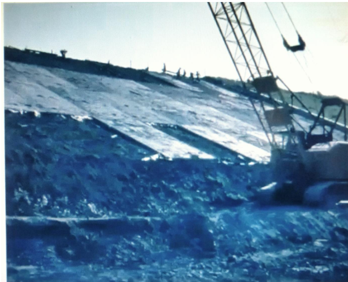
Fig 3. indicates the construction sequence (top down) for casting the spillway panels and the unavoidable damage to structure at the foot of the dam done by the crane. The earth fill of the shoulder exposed here contains a surprisingly high proportion of big stones which provide excellent routes for erosion channels to develop. (Photo ex July seminars)
