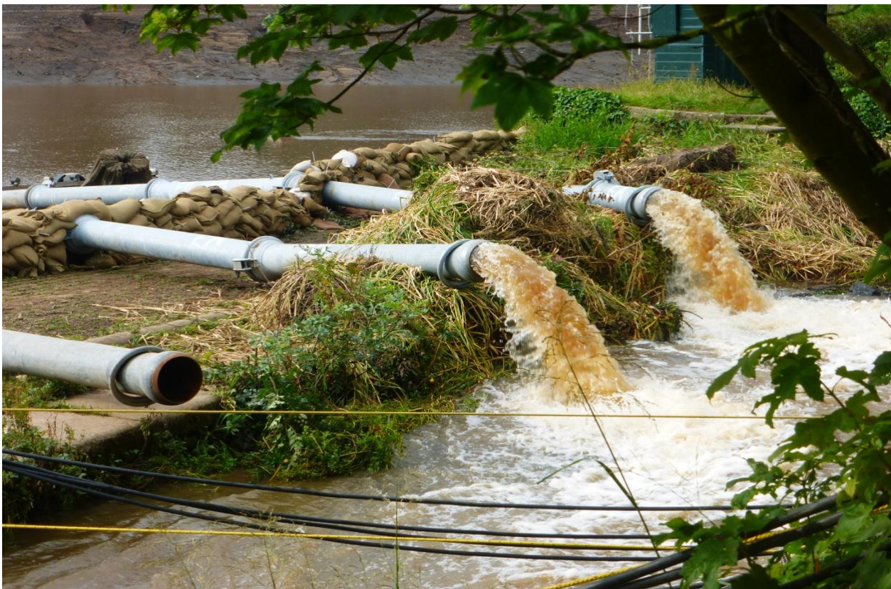
Photo 6. Emergency pumping arrangements further illustrate this deficiency as described.
