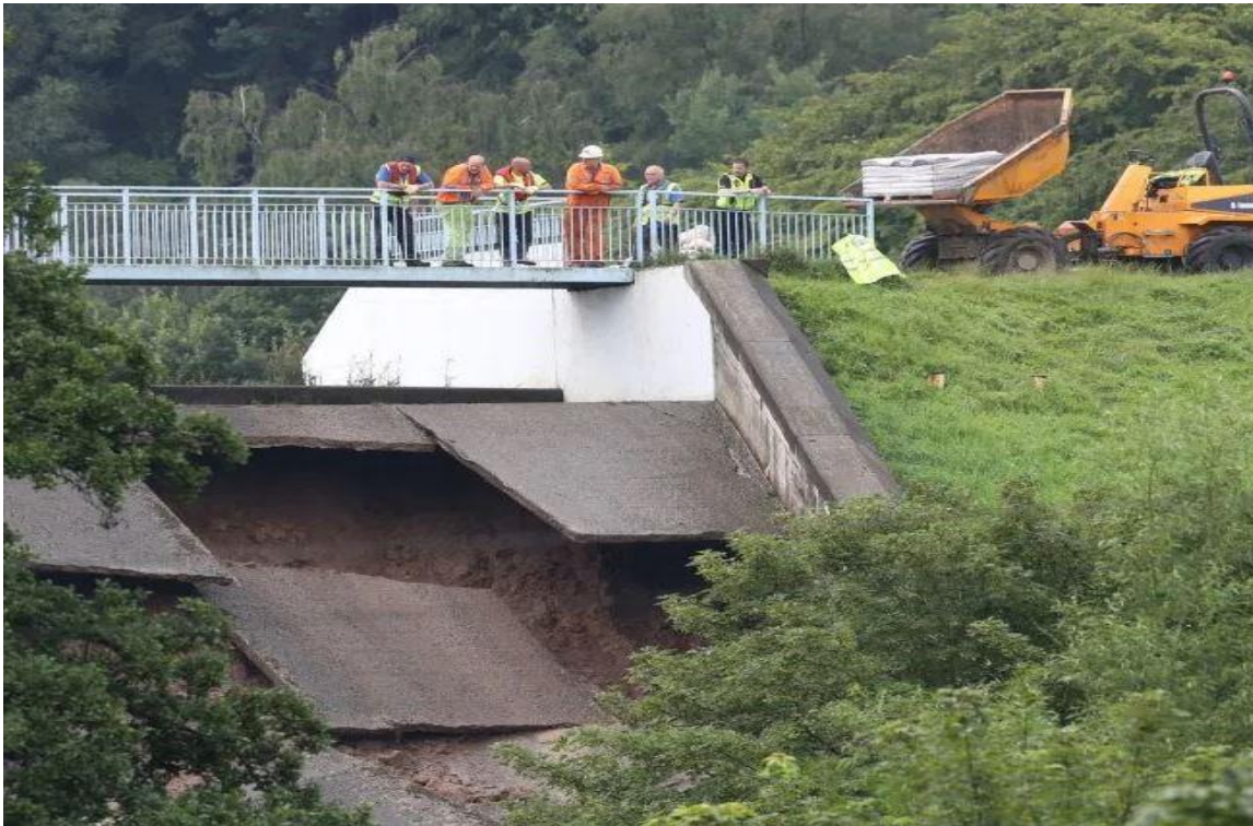
Photo 13 (above). A early picture taken not long after the flow has stopped. There is a significant large cavity under the RH spillway panel where the wall footing was undermined.
