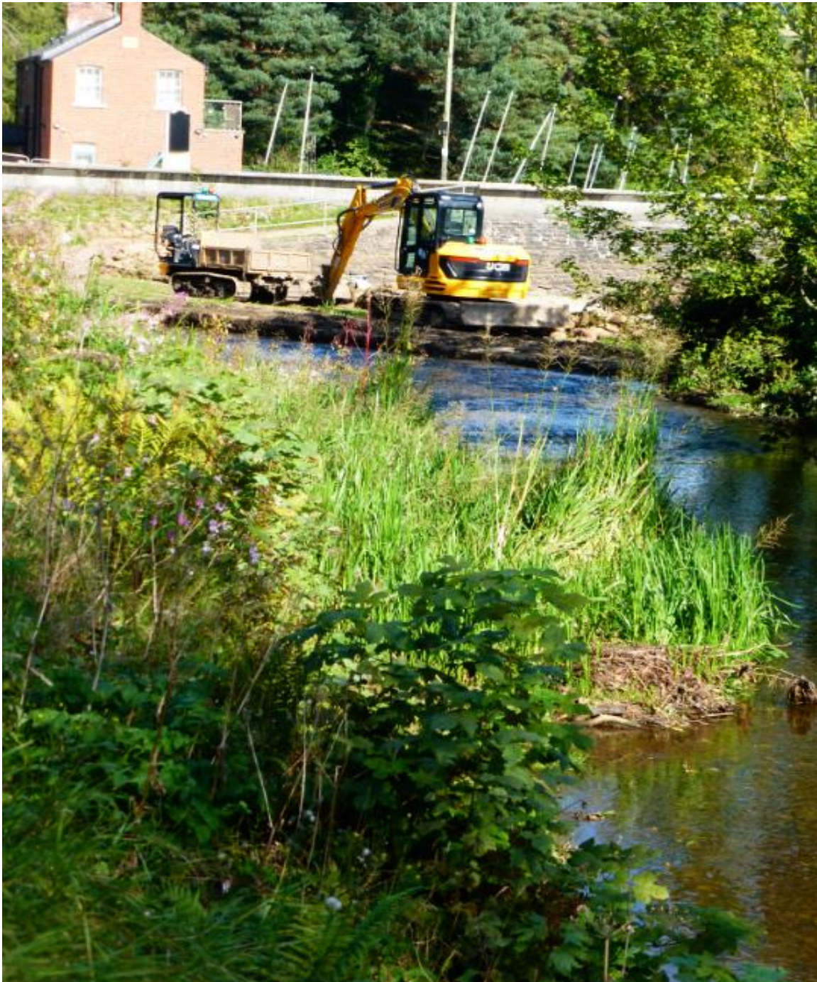
Photo 3 : A typical mud bank and weed obstruction in the Bypass..
