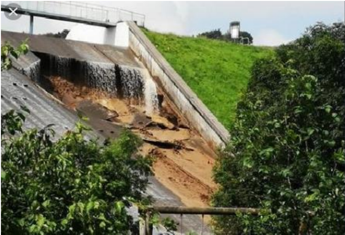
Photo 11(above) : More panels have dropped and the appalling inadequate footings of the side walls are exposed.
