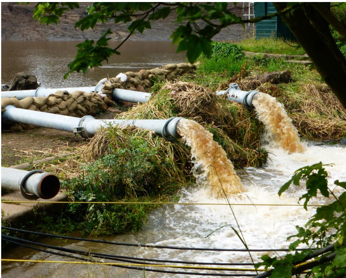
Photo 2: Pumping out the reservoir, showing a pile of weeds and mud obstructions which had to be removed initially from the Basin by the Emergency Team improve the flow when desperately trying to empty the reservoir.
