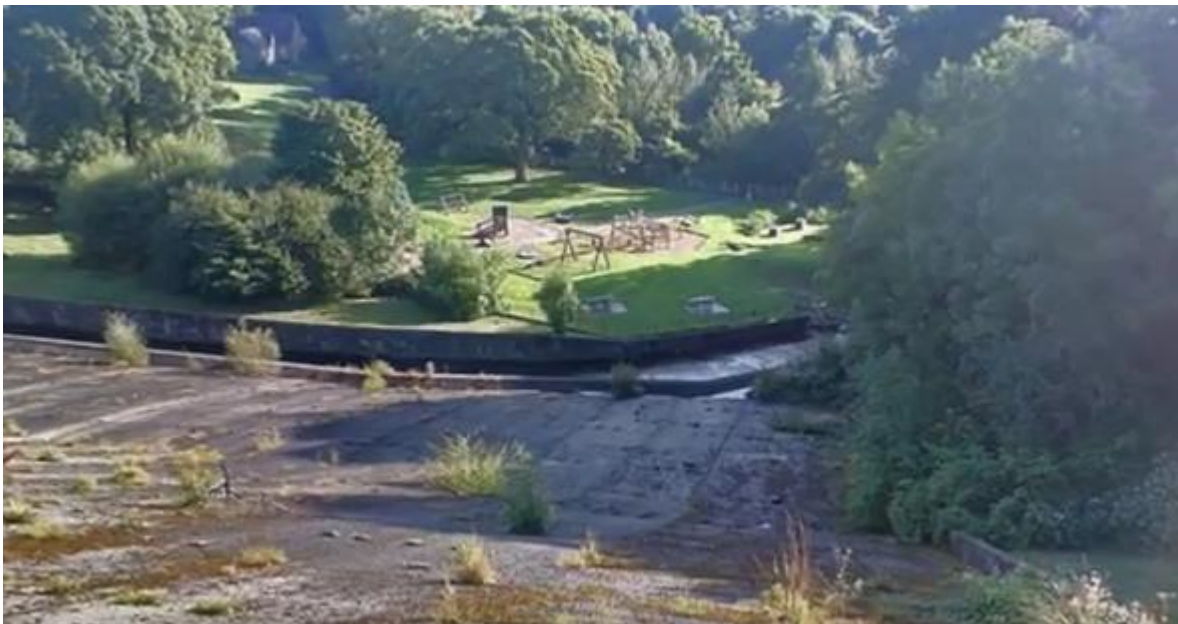
Photo 2 (above). A variety of weeds and shrubs have always flourished in the unsealed margins of the 170 panels of the Spillway and Apron, therefore the roots can easily find water underneath the panels. Mosses and lichens grow well on the decaying rough concrete surface.
