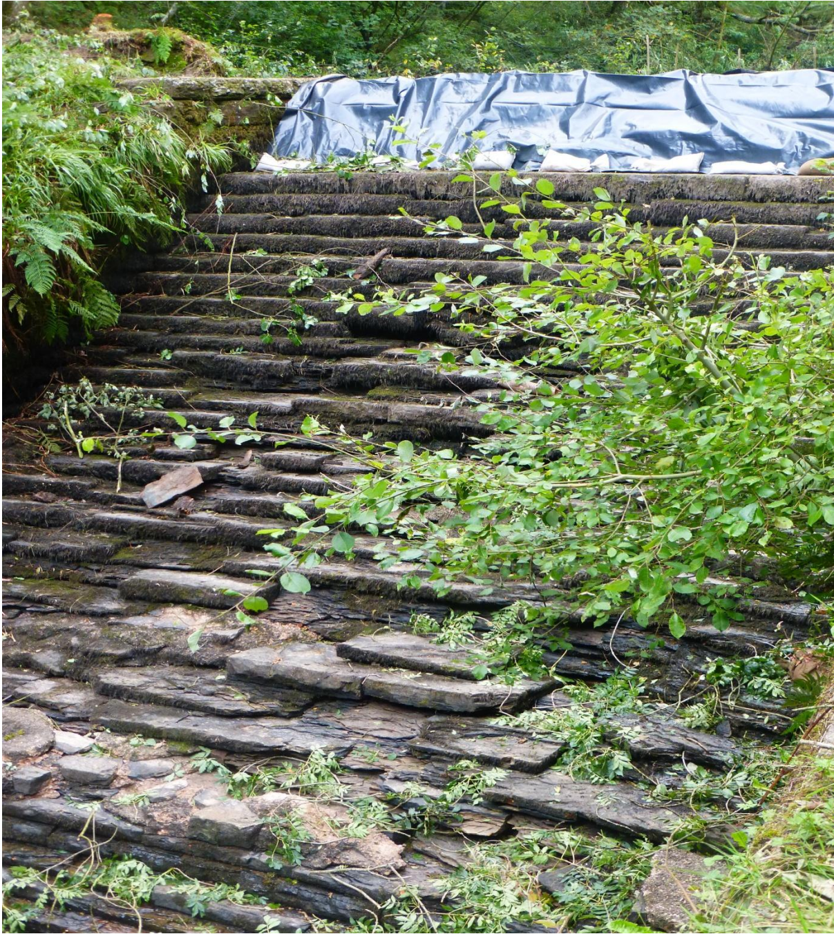
Photo 5: The downstream view of the weir itself after the incident in Aug 2019 showing the accumulation of 180 years of damage and neglect.
