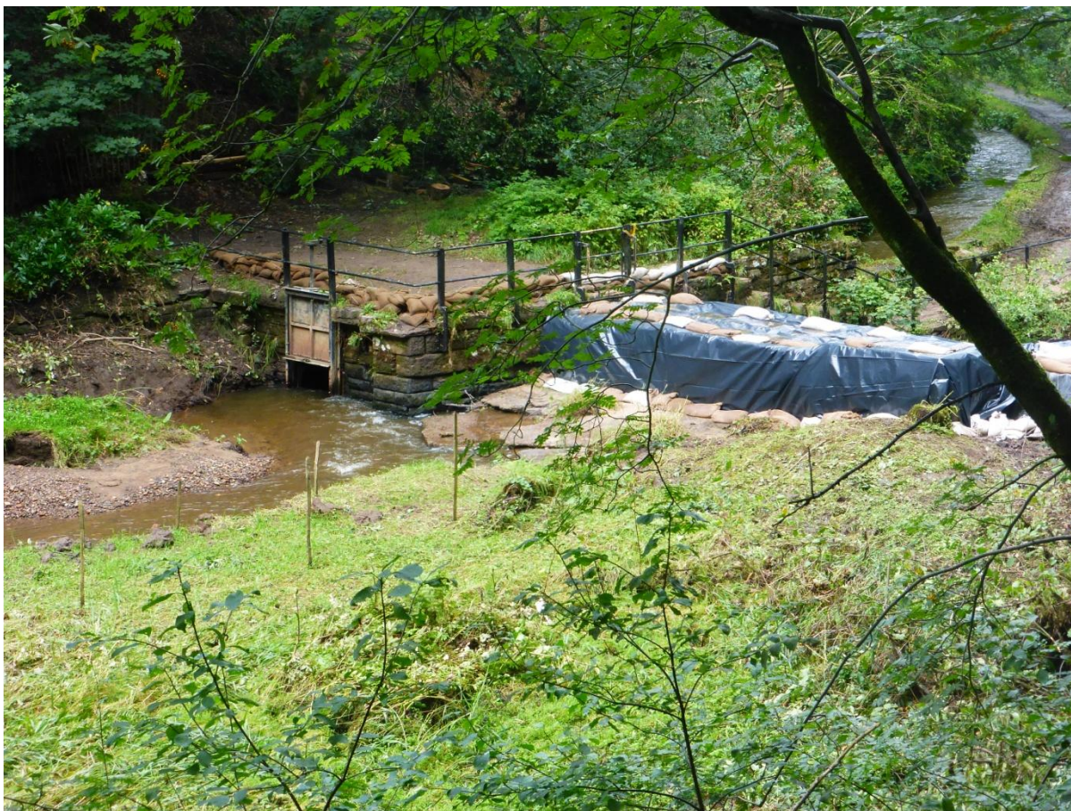
Photo 4 : The upstream view of the Weir and Bypass Gate illustrates the whole arrangement at the weir, the obstruction of the mud bank, also showing the Bypass channel running towards the Convergence Basin ( a mile away) by the footpath (top Right) .
