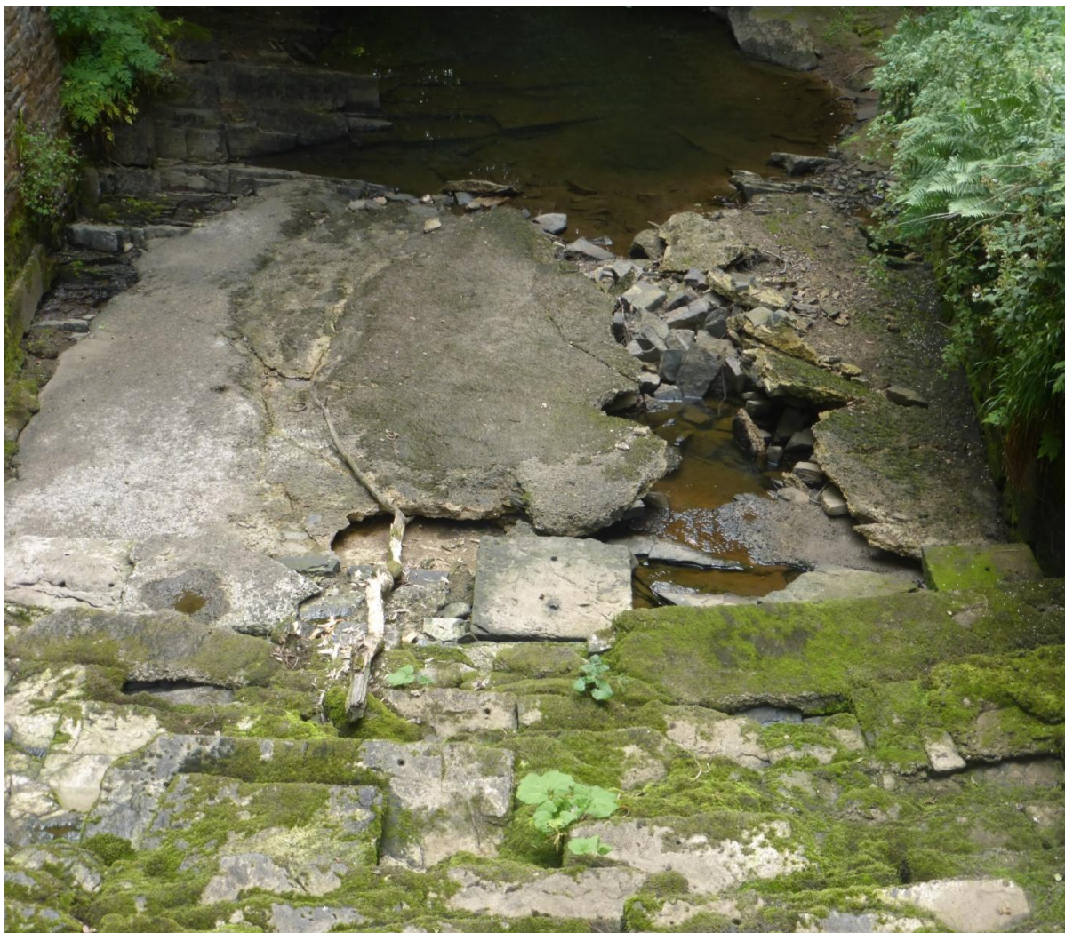
Photo 6: This was the state of the bottom of the weir in July 2017 showing failed historic attempts to prevent the undermining and destabilising the weir base by crude concrete infill repairs superimposed on each other. By Aug 2019 these repairs have already failed, previously attacked and broken by the power of successive floods, as photo 7 shows.
