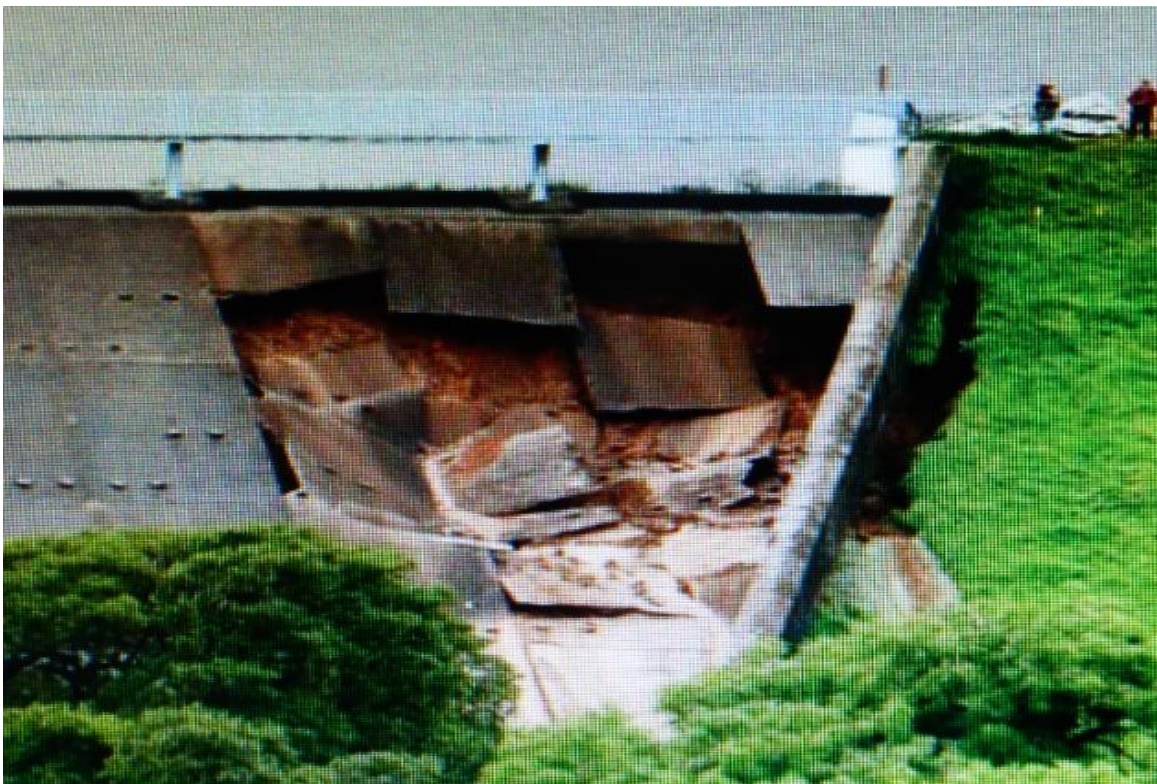
Photo 12 (above): The Gap 2 spillway panels have now both snapped in half and fallen into the empty void. Thin sheets of concrete without metal reinforcement and weakened by minimal water in the concrete mixture when cast are especially brittle and can easily be snapped.
