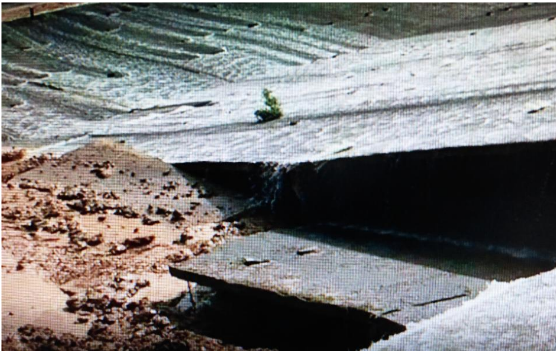
Photo 10 (above) : As in Photo 9 but taken from the footway looking down, showing the big empty cavity underneath adjacent spillway panels to the right where more of the clay core has been excavated which will lead to the further collapse seen in photo 11.
