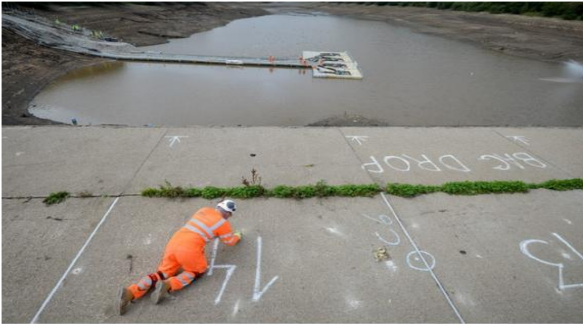
Photo 18 (above). Grouting the Apron ? All the middle Apron panels have been given numbers. There are 2 Apron panels spanning each Gap, (except that Gap 1 has 3 apron panels).
