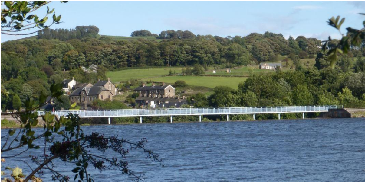
Photo 1 (above). The footway has 9 support legs (one hidden by the bush) plus 2 supporting abutments therefore there are 10 gaps under the footbridge. For this survey these gaps will be called Gaps 1-10 numbered from the left in this picture. The damage occurred in the middle of the dam on the spillway below Gap1.
